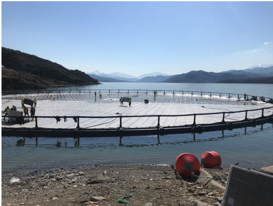
Figure 5.2. Installation of floating solar PV from Ocean Sun by the shore in Banja reservoir (photo Atle Harby).
